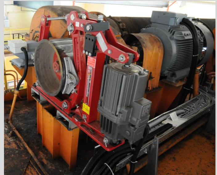
Hoist mechanism of 200/32/5 tone crane
