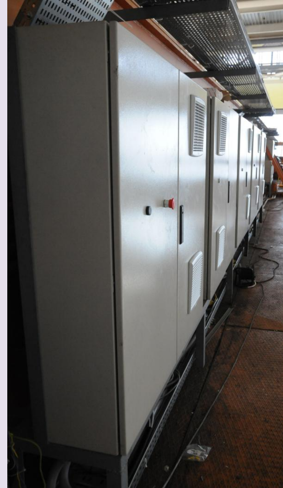
Electrical panels of crane Q=200/32/5t
