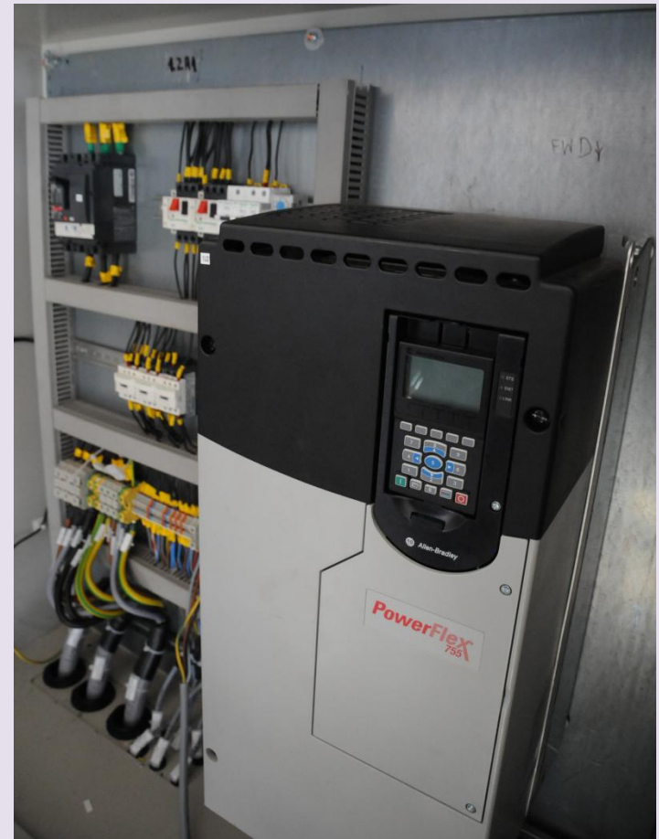
Panel for hoist control with specialized frequency inverter for heavy duty conditions.
