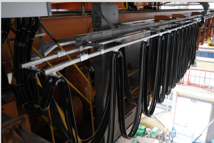
Festoon power supply of bridge crane
