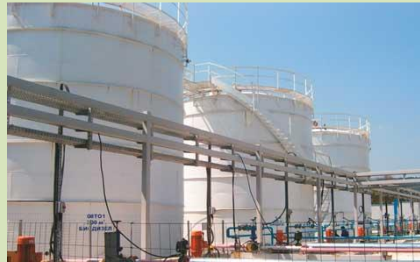
Biodiesel installation facility
