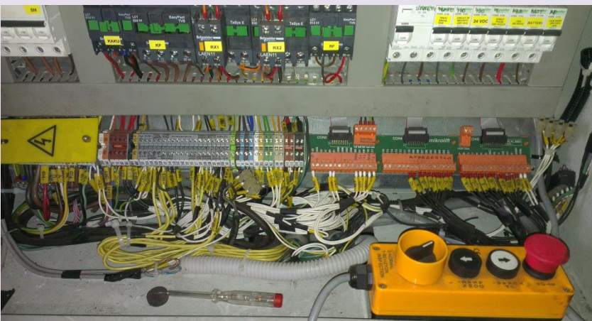
Terminals connections in electrical panels
