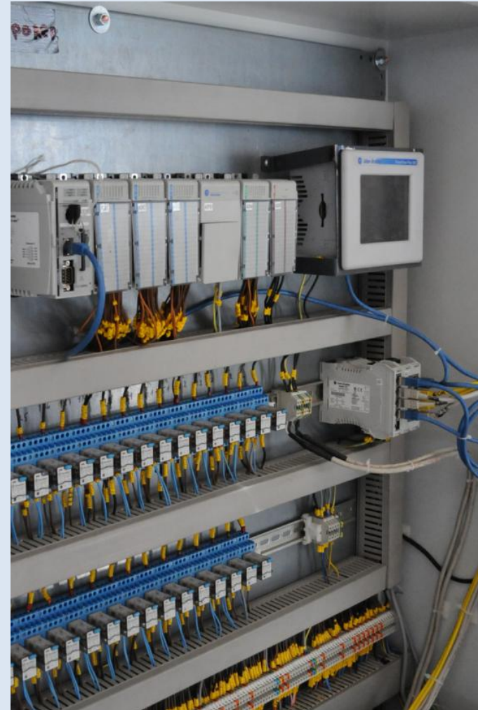
Electrical panel for control with PLC and display.
